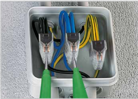
Voltage testing via separate test ports.
