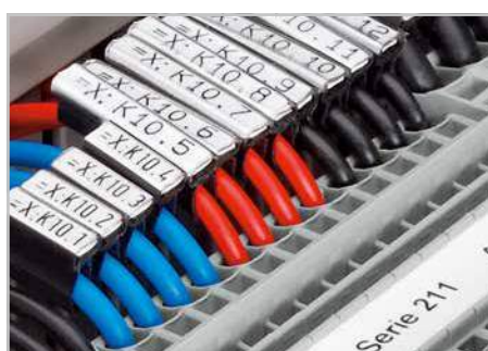
Marking conductors via marking sleeves.
